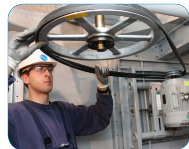
Maintenance and service expertise
